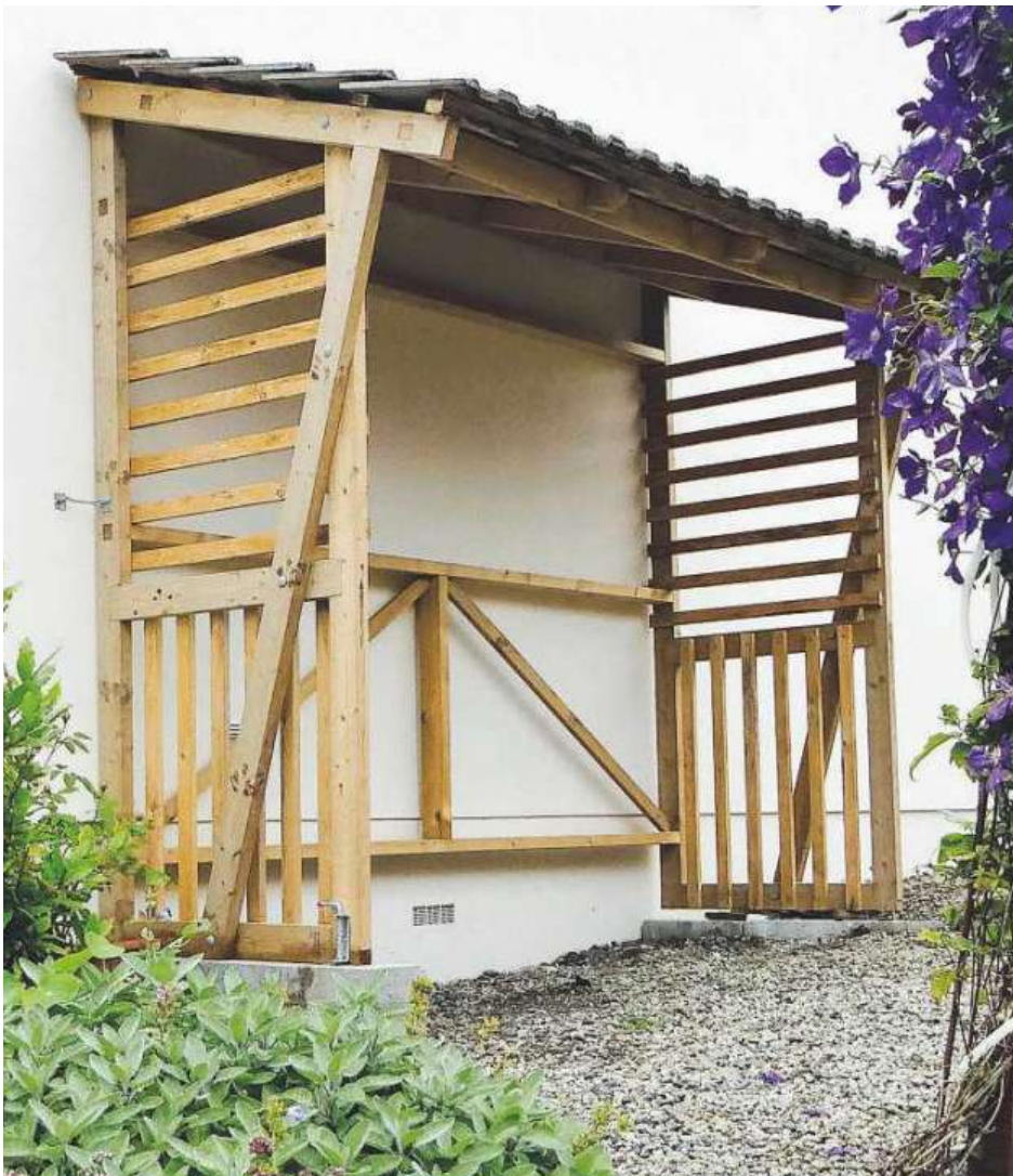
Please excuse the foundation block on the right which ended up lower than the one on the left. I was hasty
